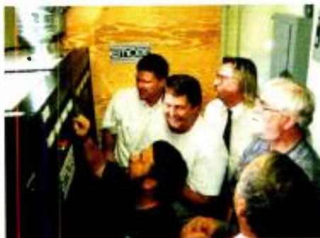
Emcee Chief Engineer Bob Nash (far right, with glasses) and other engineers watch as WITF-TV Chief Engineer Larry Winemiller (in dark shirt) switches on the station's Emcee 25 kw digital transmitter.
