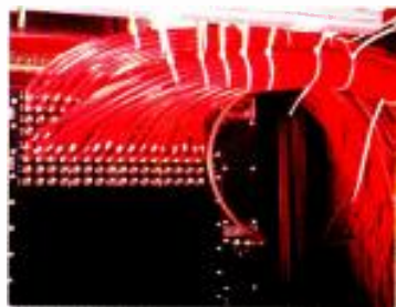
WLVI-TV has installed Mohawk/CDT Spectrum coax cable.
