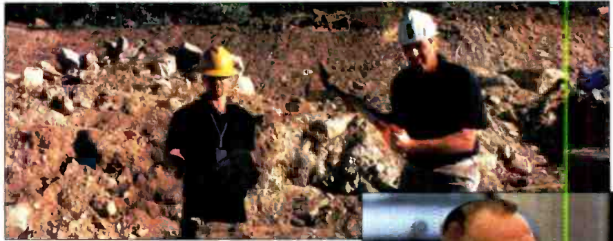
Cox's Jim Robbins (r) and field service leader Andrew McCarthy at work on Cox's master telecommunications center in Rhode Island.
