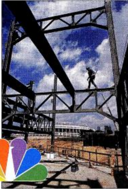
Construction on Olympic Stadium is well under way, as are advertising sales.
