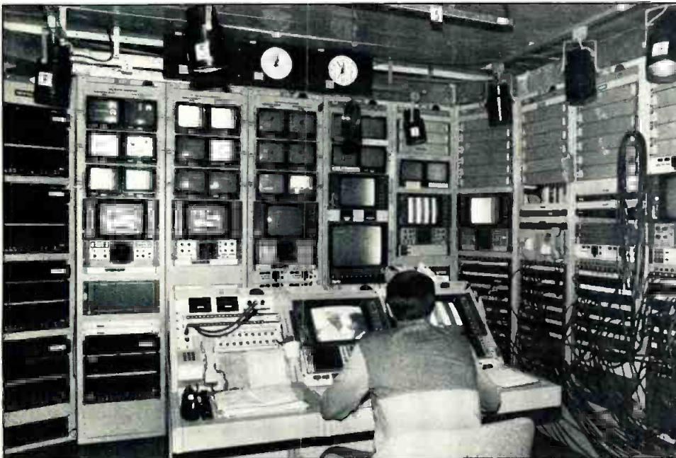
ABC's Olympic control room
