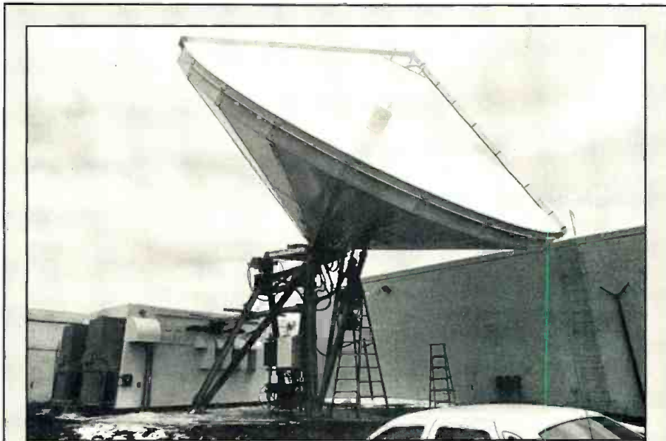
Satellite newcomer. Meadowlands Communications Inc., which plans to offer a wide range of satellite transmission services, is moving ahead with plans to establish a network of satellite earth stations in 26 cities.
