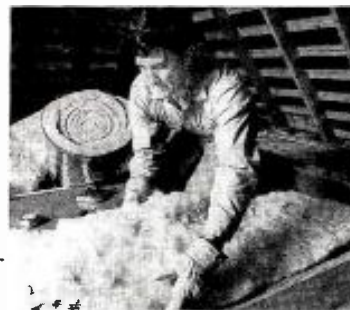
Conservation around the home could cut energy consumption by 14%.
