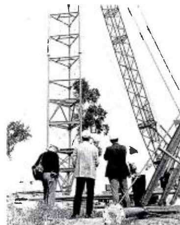
Room for all. Stainless Inc., North Wales, Pa., is fabricating a new 2,000-foot tower for KCRG-TV Cedar Rapids-Waterloo, Iowa, which the station will share with the Iowa Educational Broadcasting Network, and University of Northern Iowa's KUNI-(FM) Cedar Falls. International Tower Systems, Menomonee Falls, Wis., has contract for erecting the tower. The station's former tower collapsed Oct. 3, 1973, while workmen were modifying it, killing five persons. The first section of the new antenna is shown being hoisted into place. Completion is expected by late October.
