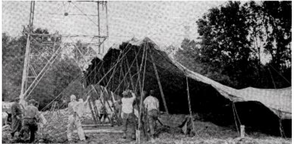
IN KEEPING with the tradition that "the show must go on"—this particular one on Oct. 27—workmen erect a tent which will allow WTVW's studio and transmitter foundation to be constructed despite interference from the elements.
