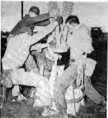
TOWER of KWTV (TV) Oklahoma City, which was completed Dec. 5, had its basic supporting structure anchored just two days earlier. The station was scheduled to start regular programming, as a CBS-TV affiliate, yesterday (Sunday) on ch. 9.
