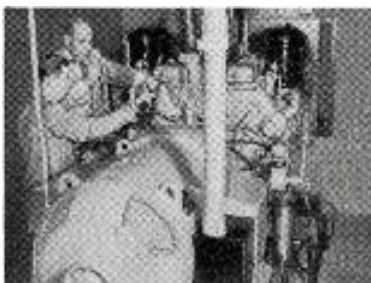
WJR—Detroit, Michigan, uses 200 kw. GM Diesel generator set as stand-by power for 50,000-watt transmitter. Compactness of unit permitted installation in garage adjoining transmitter building—eliminating cost of a specially designed building.
