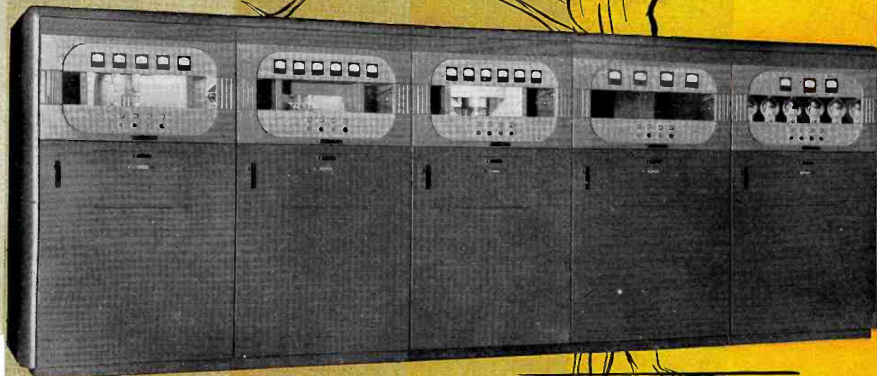
Collins 736A-1 50,000 watt FM transmitter
