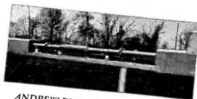
ANDREW FM-AM isolation section with cover removed, revealing two 3/8" FM transmission lines and expansion joints.
