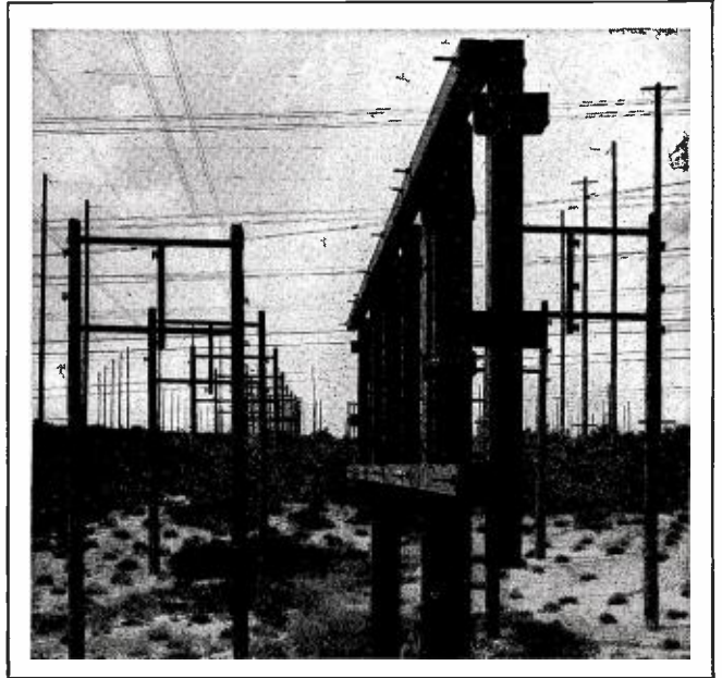
At the Riverhead, Long Island, receiving station of RCA Communications are scores of antennas. This is the point of reception of European features that are heard on hundreds of American radio stations.
