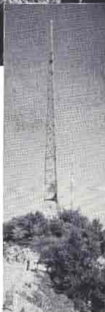
Designed for a 30-yr. wind load with 7" of radial ice, this 200' Ideco tower for KTTV atop Mt. Wilson supports a 6 bay channel 11 antenna.
