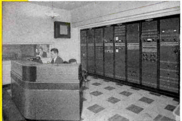
KCRG Control Room — Special speech equipment installations are a specialty of Collins. The equipment shown uses standard amplifiers and panels, thus taking advantage of price savings in mass production.
