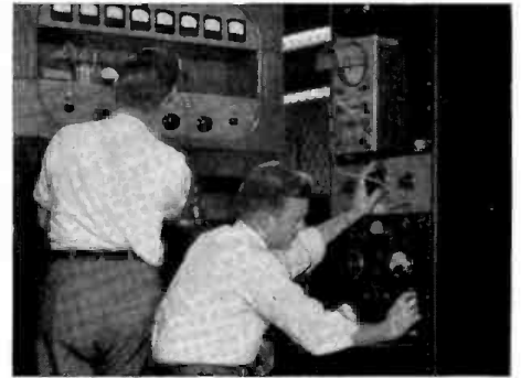
Taking performance data on a 1 kilowatt broadcast transmitter. Final test of the completed product using the latest and best apparatus known. This assures the finest overall performance.
