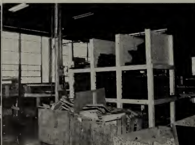
Large rack of covered rails stand at the ready after slate is installed.
