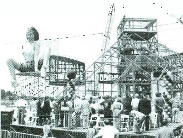
Rock And Roll Hall Of Fame and Museum board members, officials, and guests look on as the structure that will house the hall is topped off. The final beam is seen at the top right of the structure. At left is the inflatable "Ruby" from the Rolling Stones' Steel Wheels tour. The Hall Of Fame is set to open on Labor Day 1995.
