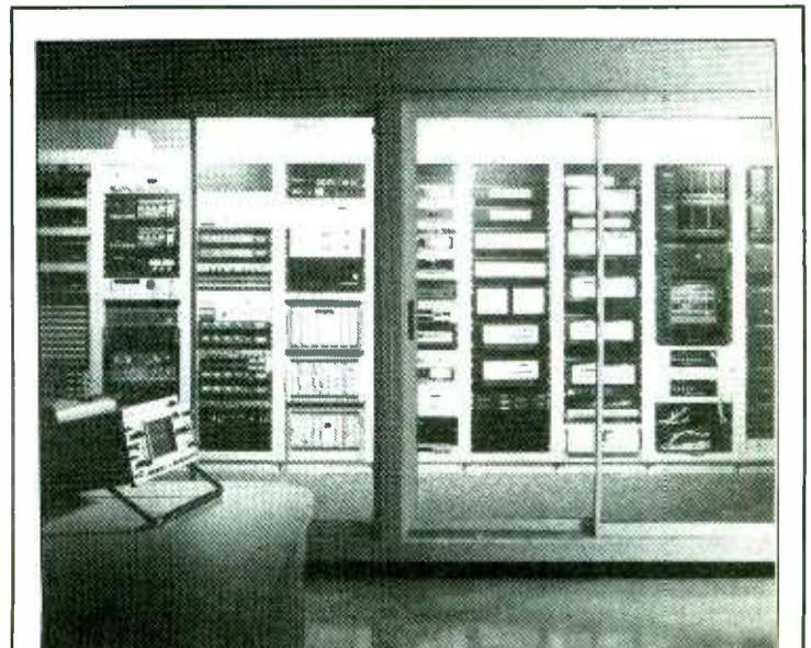
WKHX's well-organized terminal room.
