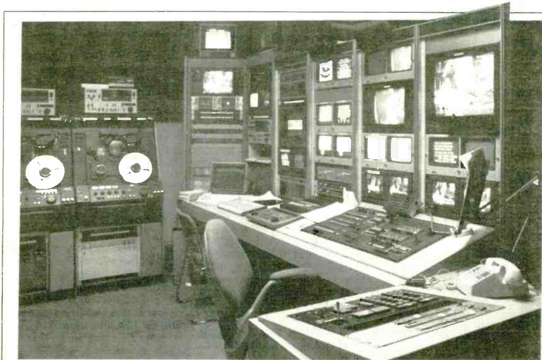
The state-of-the-art Q-Zoo Tube control room, which was installed just down the hall from the air studio.
