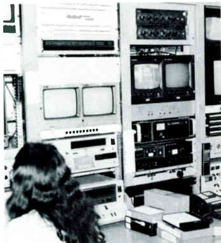
The TV 10 control room.
