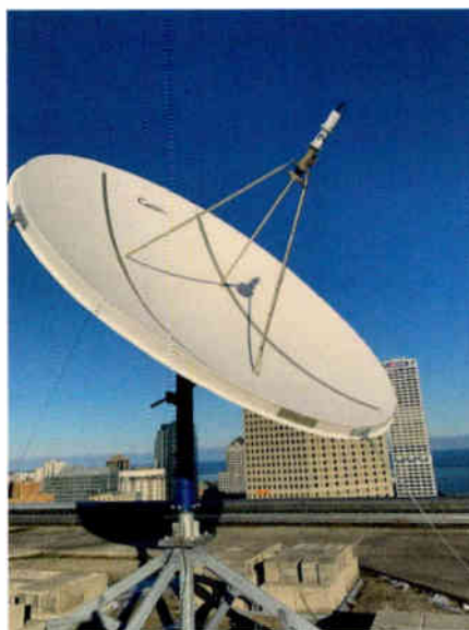
Above Comtech dish on roof of WUWM Radio in Milwaukee.
