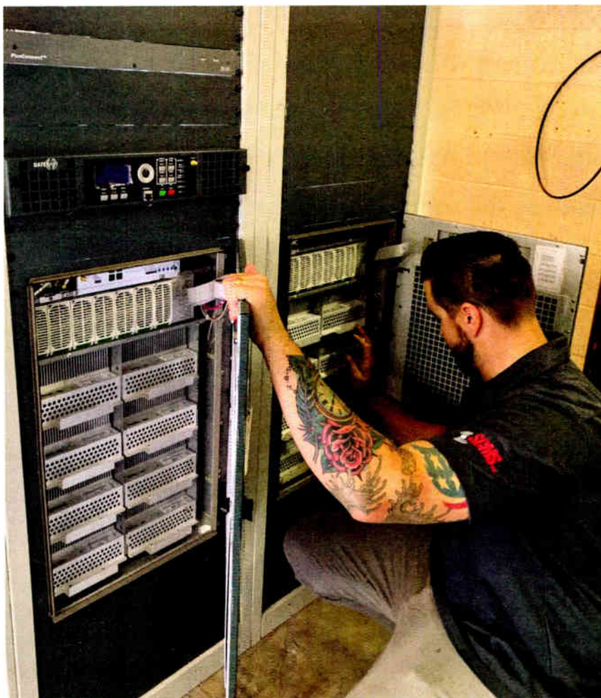
On-site at KZZO(FM), installing a GatesAir FAX20 transmitter.
