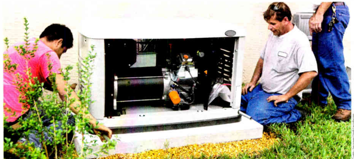
Generators must be tested under load ... all the loads!
