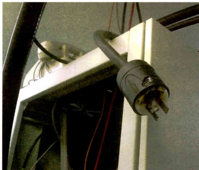
Fig. 1: Heat from loose wiring connections points to the source of the failure. The blackened plug is a clue.
