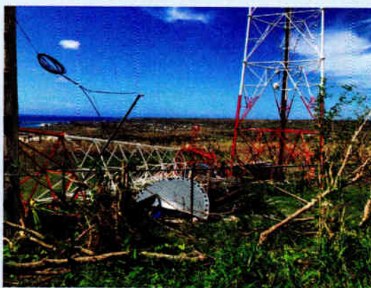
Destroyed telephone service tower on Tinian.
