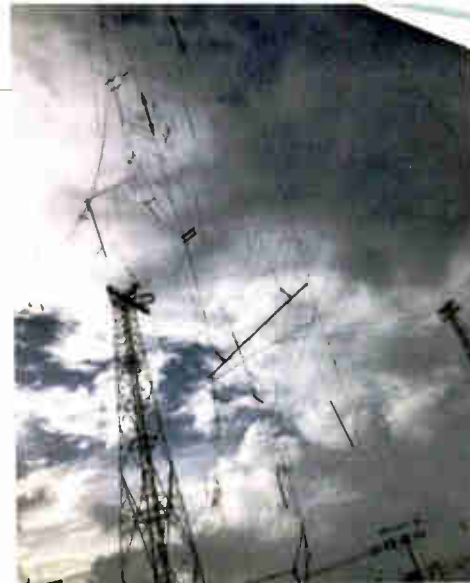
Above: Damage to antenna feed line on Saipan
