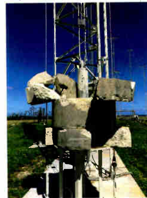
Below: Damage to antenna counterweight on Tinian
