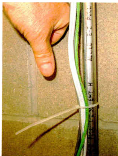
Fig. 1: Thumbs down on illegal wiring.
