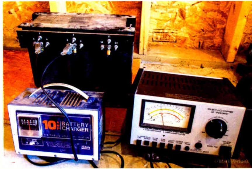
Fig. 1: Heating transformer coils with a battery charger and variable AC power supply.
