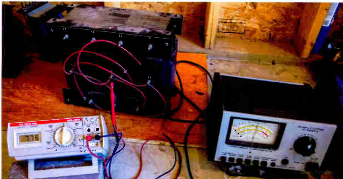
Fig. 2: Testing high voltage using a variable AC power supply on a primary winding.
