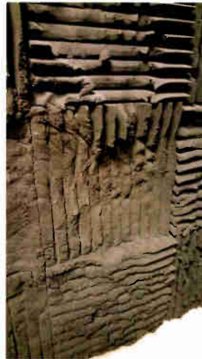
Fig. 2: Foam panels deteriorate. Depending on their age, they may also pose a fire hazard.
