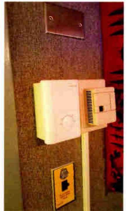
Fig. 4: Cut the foam away from light switches or thermostats to reduce damage from hands.
