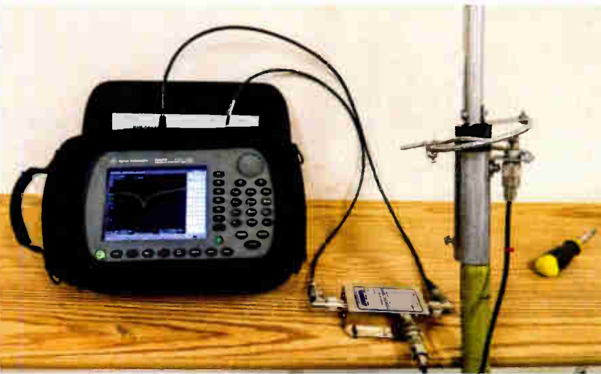
Fig. 6: A spectrum analyzer with return loss bridge measuring and tuning a remote pickup antenna for low reflected power.
