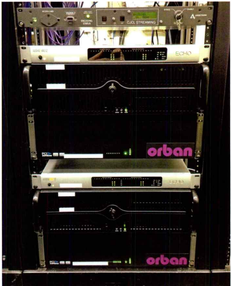
A pair of easily identified Orban OptiEXP expansion chassis at the Rogers Broadcasting Toronto facility.
