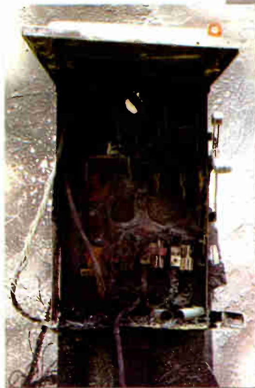
Fig 2: There's not much left after this fire.
