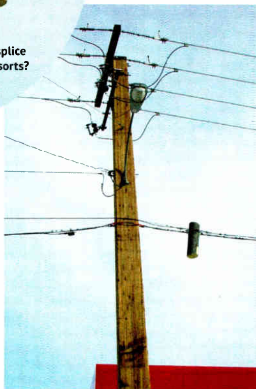
Fig. 3: A chunk of “old pole” remains as the cables must be remounted.
