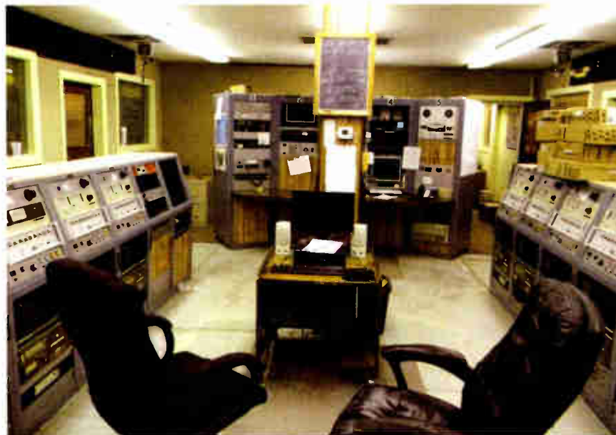
Master control of WYFR, now WRMI, where all of the audio is distributed and computers control transmitters, frequency and antenna changes.
