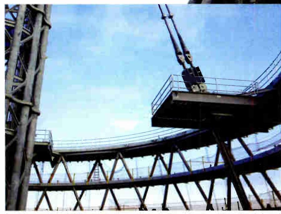
Left: A closeup of one of the four spire guy sets. Phillystran supplied eight aramid fiber high-performance tower guy assemblies, each approximately 100 feet long and 6 inches in diameter, to support the mast. These custom assemblies are the largest Phillystran tower guys ever assembled and have a rated break strength over 1.7 million pounds.
