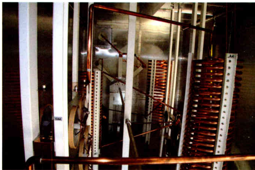
The Antenna Tuning Unit at Burg
