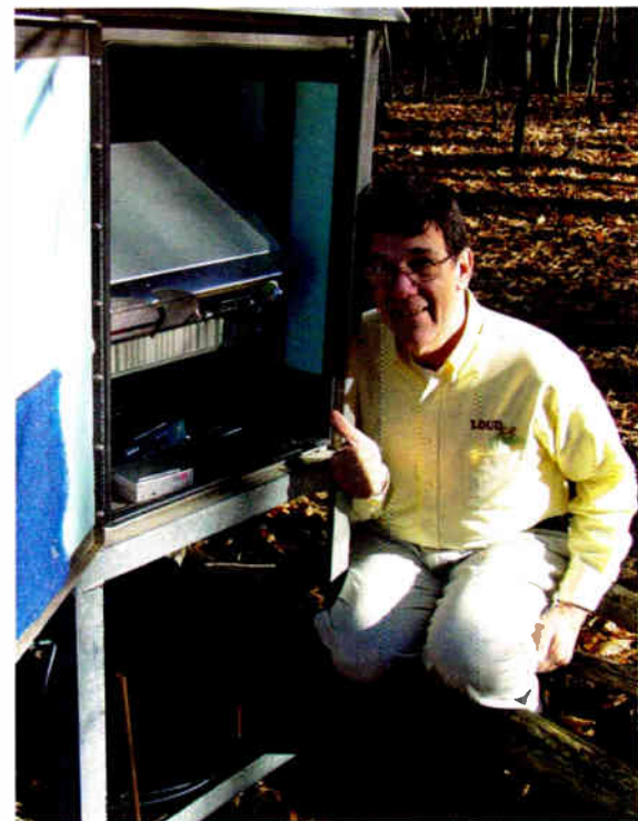
The author and his transmitter box. Note the steeply angled Elenos transmitter: Its exhaust fans on the backplane are at the top of the box to vent excess heat.
