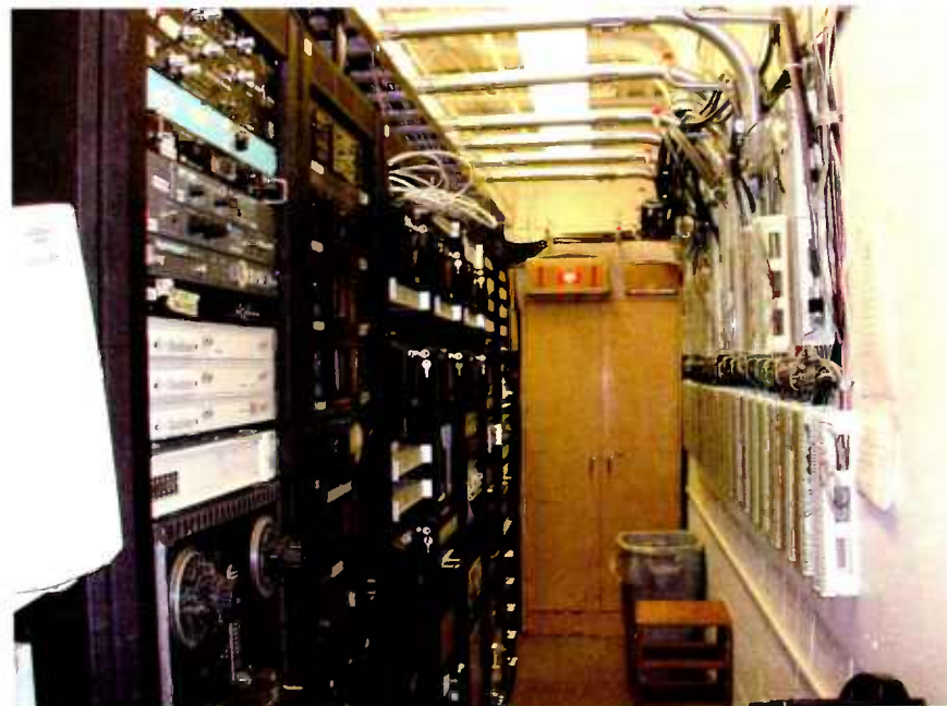
Use the list of assets to be conveyed as a checklist as you inspect the equipment.
