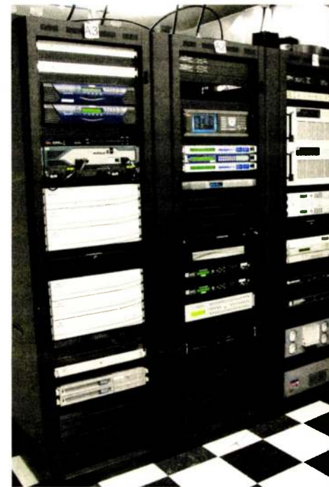
Equipment racks at the Indianapolis uplink.
