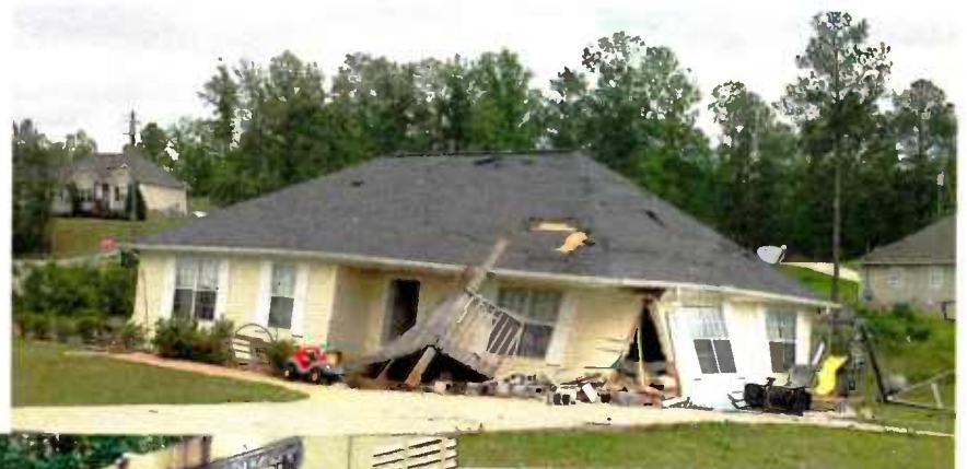
Our chief engineer's house sustained only minor damage, but this neighbor was not so fortunate.
