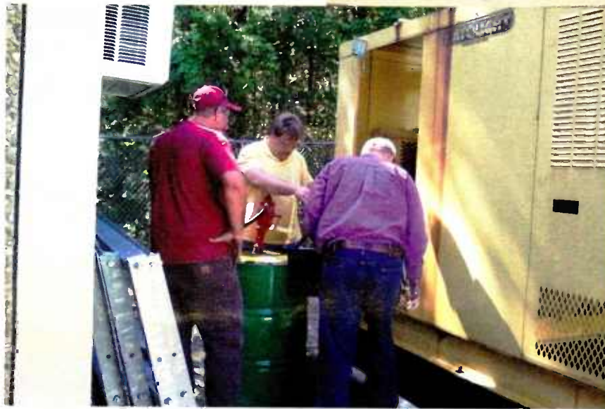
Refueling the generator at the Cullman site from a 55-gallon drum was part of the daily grind until the power came back on.
