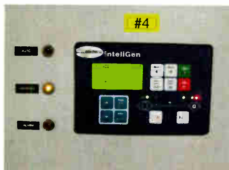
Fig. 4: The Inteligen control panel after installation.
