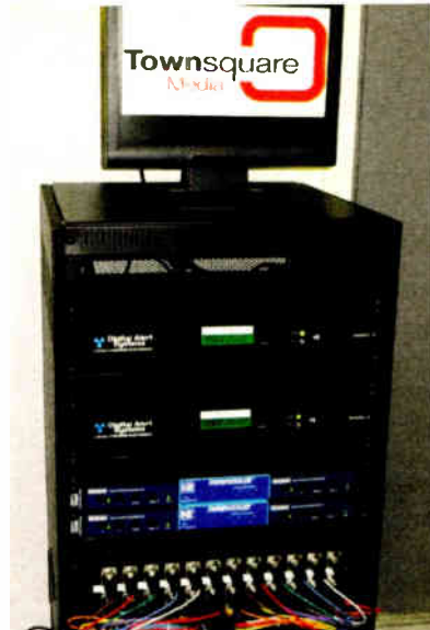
EAS equipment is part of this gear rack at Townsquare Media.
