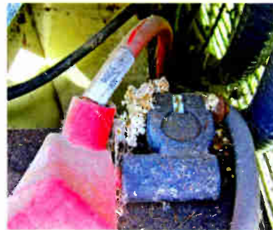
A corroded battery terminal. Often the positive battery terminal corrodes first.
