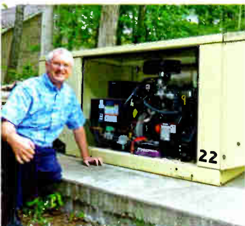
Mark Persons. 'Gensets are a serious maintenance item.'
