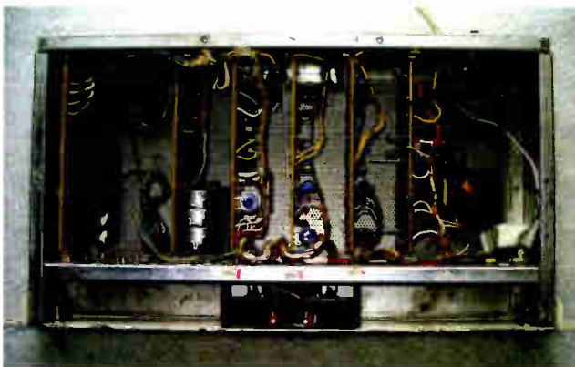
The classic 400 series layout, with PCBs in a card cage configuration interconnected with cable harnesses.
