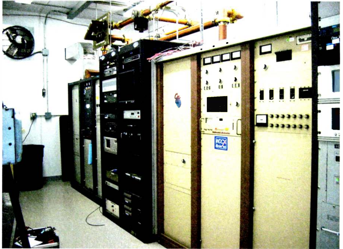
Identify vulnerabilities and don't even think about deferring maintenance on that aux transmitter!
