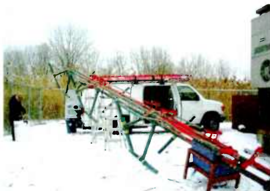
When it snows, it pours. This FM antenna coincidentally failed at the same time as an audio processor and a whole-site UPS unit.
