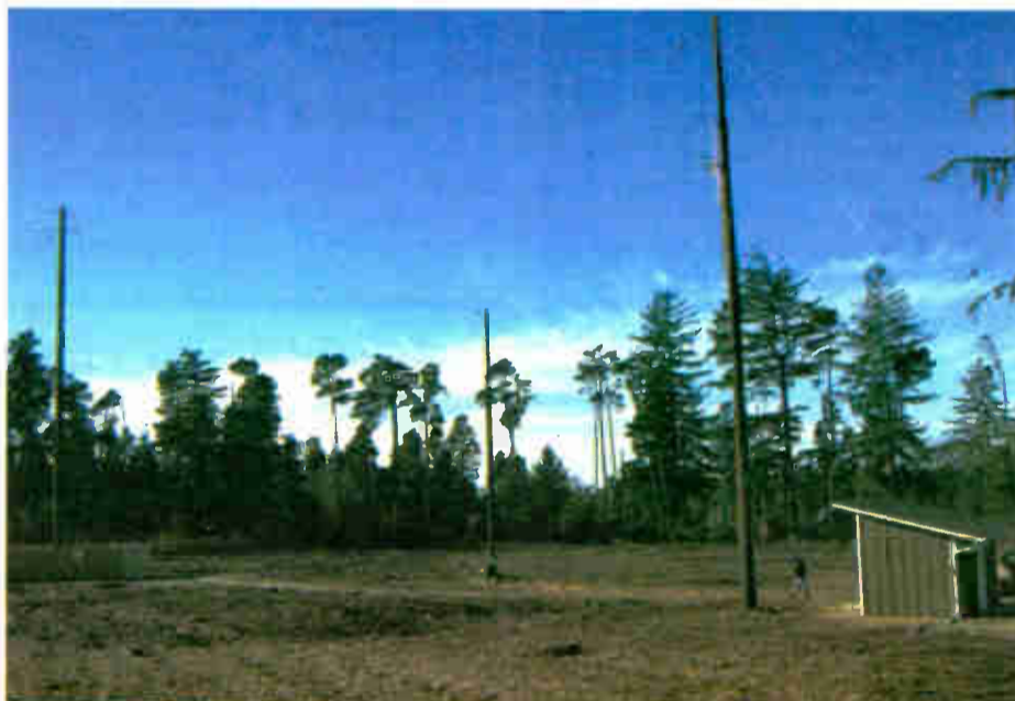
Fig. 3: You've heard of tower farms; this is a phone pole farm. A view of the KCST KinStar antenna, with the center feed at the left, three of the five support poles shown, and the transmitter building on the right with the STL dish installed on the pole closest to the transmitter building.
