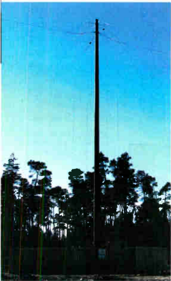
Kintronic will discuss the first installation of its low-profile KinStar antenna at KCST(AM) in Florence, Ore.
