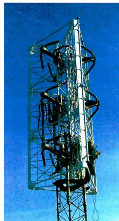
Myron Fanton of ERI will discuss the case study of a multi-station combined analog/digital antenna on a building top. Shown, a worker (lower right) prepares the structure for another bay.
