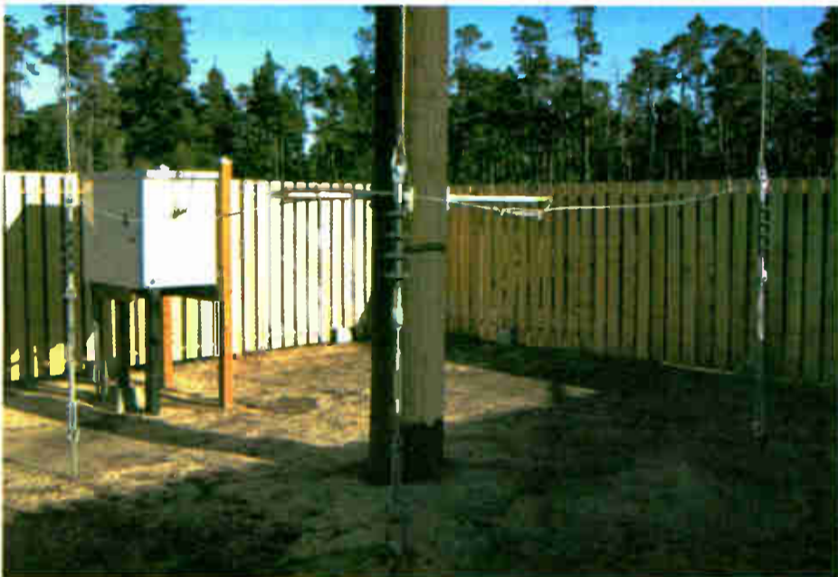
Fig. 2: This is the feedpoint of the KCST antenna, showing three of the four insulated vertical elements with the associated commoning ring and the Kintronic Labs Model LTU-1B-1600 antenna matching unit.
