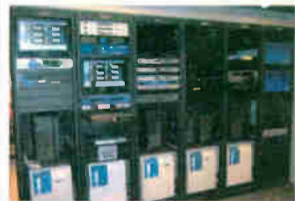
Racks at New Hampshire Public Radio
