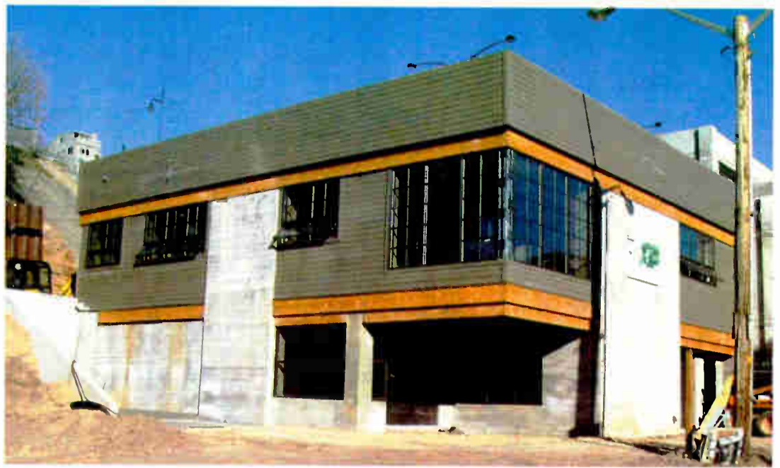
This is the exterior of the nearly completed facility; the air studio windows are visible upper floor center.
