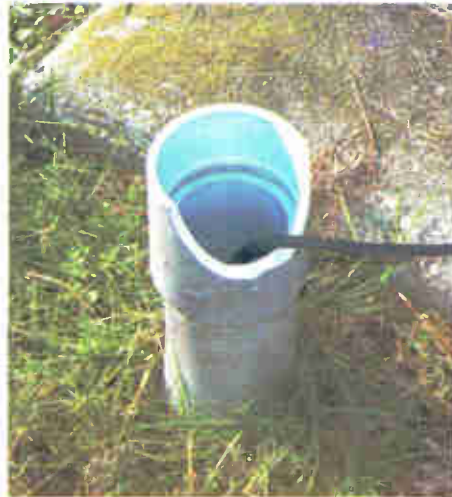
Fig. 5: Plug conduit openings like this one to keep out the elements — and worse.
