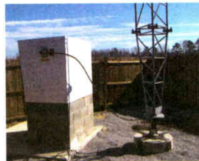
High-Power Antenna Tuning Units
