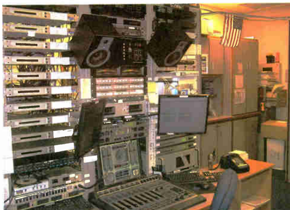
Journal Broadcast engineering rack following installation of Axia nodes.
