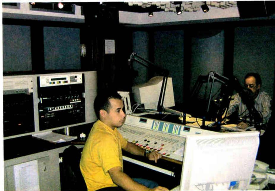
An excellent sound-absorbing scheme — panels on the walls, corner traps and diffusion blocks on the ceiling.
