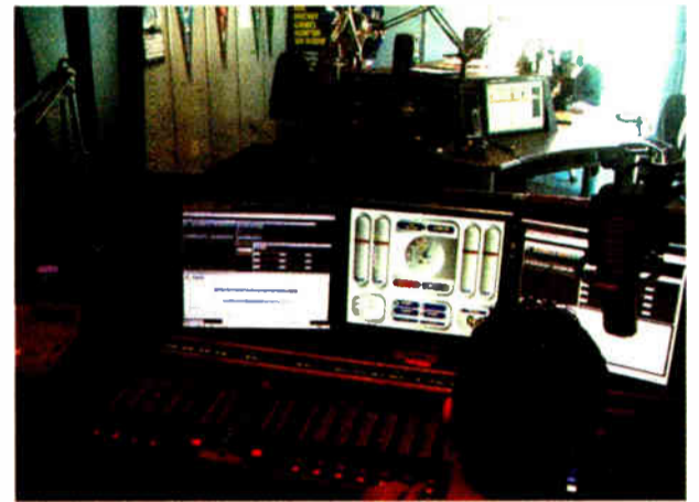
The facility boasts one of the largest Axia installations in North America.
