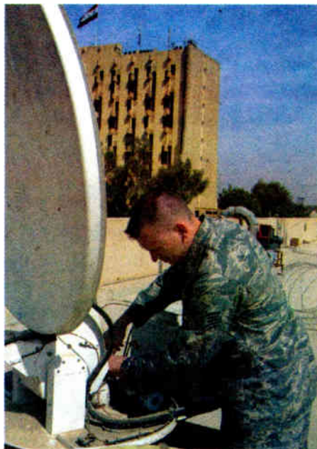
Staff Sgt. Chuck Greene works on satellite equipment on the roof of the studios in Baghdad.
