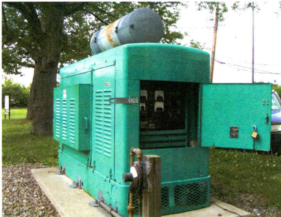
A gas generator at Clear Channel in Binghamton, N.Y.
